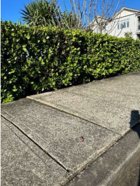
Figure 48: Lifted footpath pavers causing trips and falls (P5 AP)
