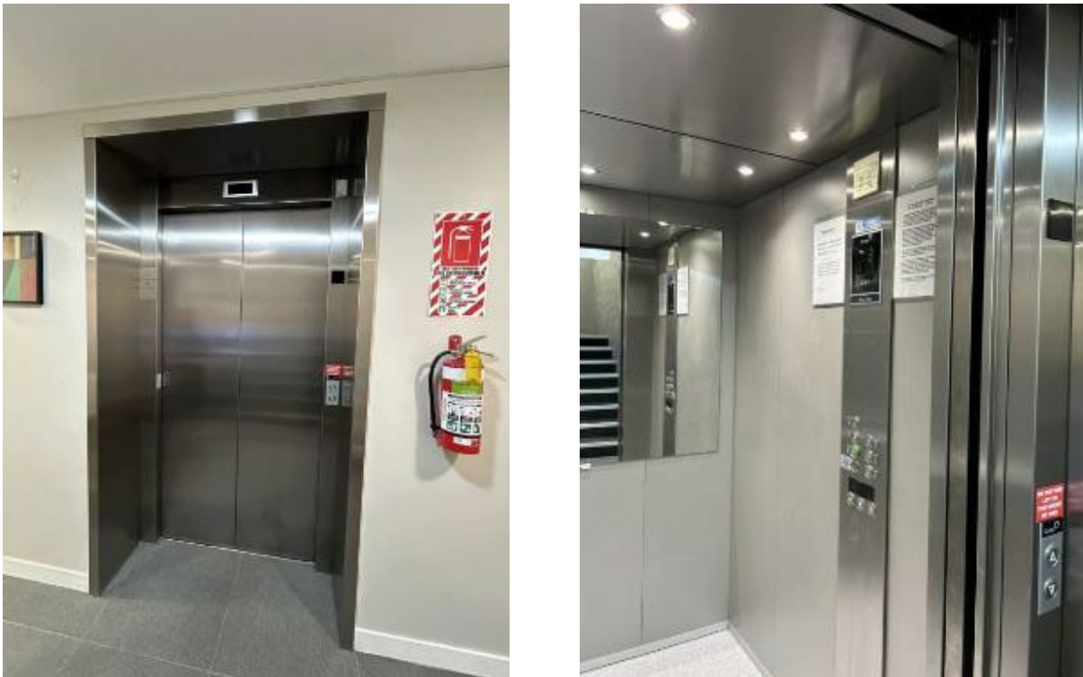
Figure 6: Exterior and interior of lift in an apartment building (P1 AP)
